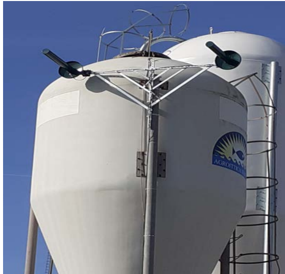
Fig. 5. Gateways and their antennas in the installation site.
