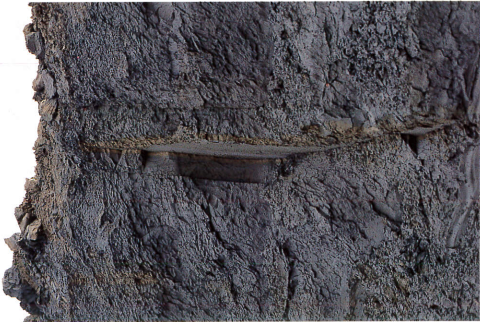
Photo 1 - Example of typical subvertical attitude of joints (Castelnuovo Berardenga quarry). In this case, as frequently happens, the fracture plane is grayish.
