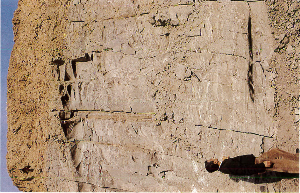
Photo 5 - Prosecution of joints as open inoxidized fracture for pressure release due to quarring.
