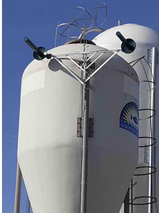
Figure 8.3: Gateways and their antennas in the installation site for setting up the LoRaWAN infrastructure monitoring offshore sea farms.
