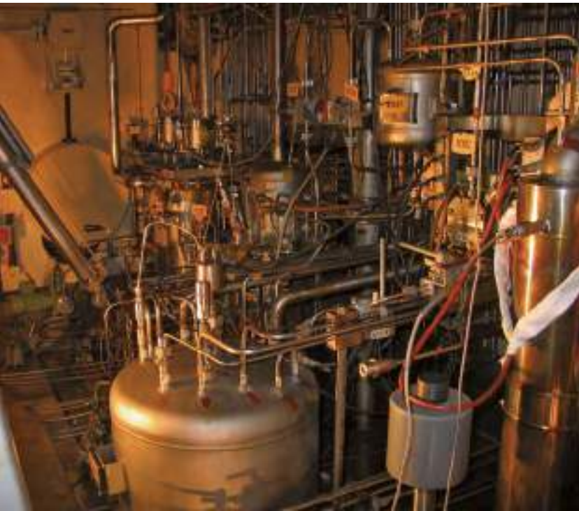
The PETRA experimental plant, which enabled the testing of slag treatment processes on high irradiance fuel.
