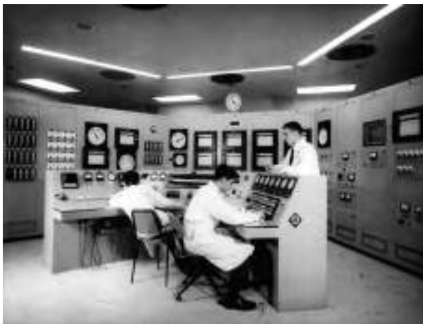
Ispra Control Room 1.
