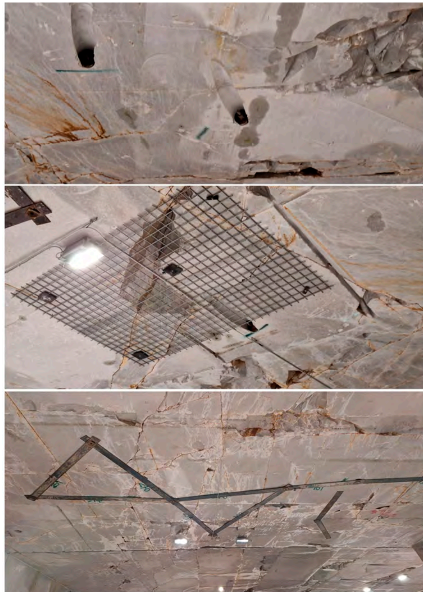
Figure 23. Examples of active supports installed in the roof of the underground tunnels.
